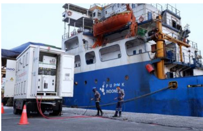
Figure6 : Shore Power Supply (Source : PELINDO Document)
