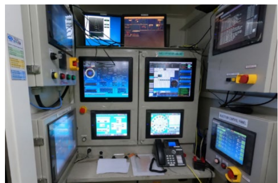
Picture-8 Central Control Room of TBM
