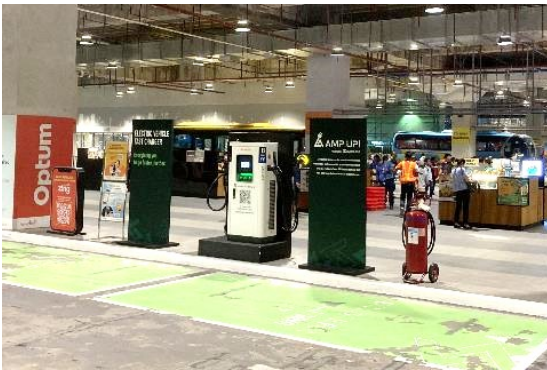
Picture-3 EV Charging Stations
